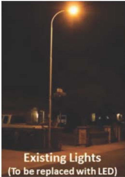
Existing 2200 Kelvin HPS
