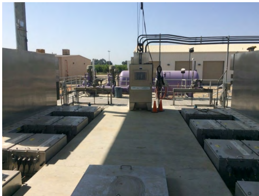
Figure 6.7 Open Channel UV Disinfection (City of Visalia)
