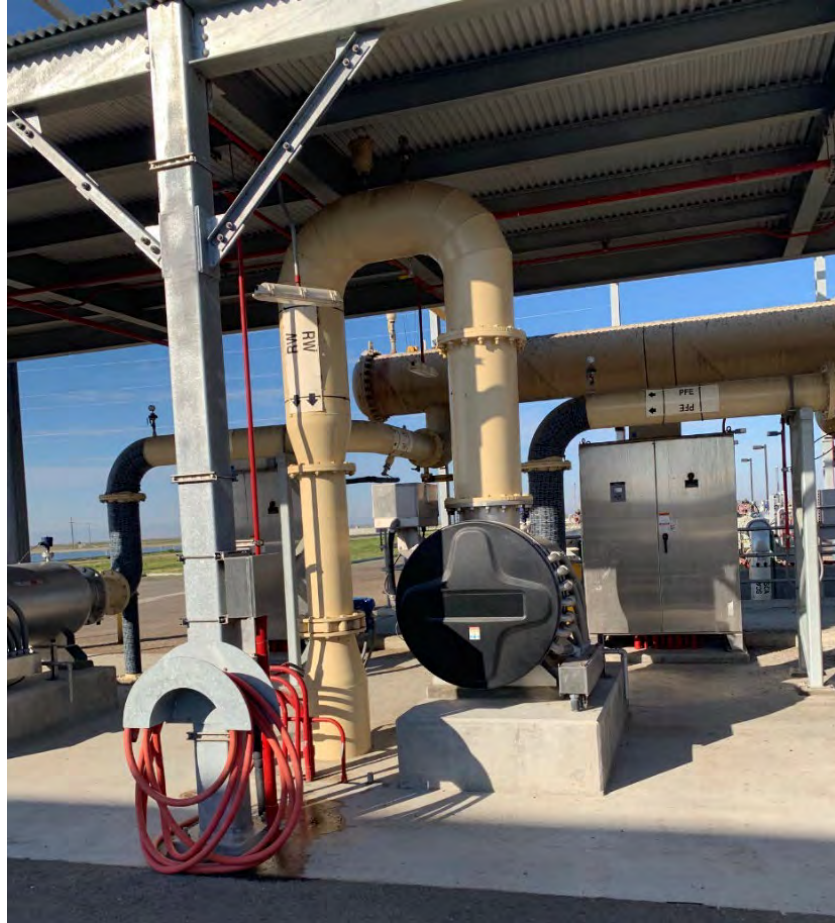
Figure 6.6 Closed-Vessel UV Disinfection (City of Fresno)
