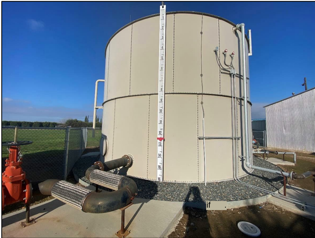
Figure 4-2 Well site at Hope Elementary. Tank in foreground.
